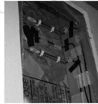
Figure 6. In-Wall Temperature and Humidity Measurement Devices, Laramie
