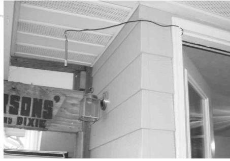
Figure 7. Location of Exterior Climate Sensor
