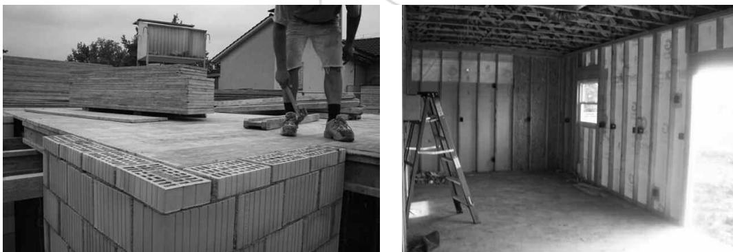
Figure 2. Swiss Masonry Walls (left) and U.S. Wood-frame Walls (right) (photos by authors)
