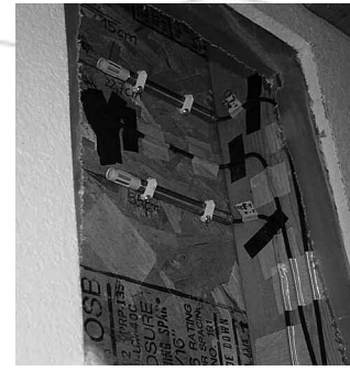
Figure 6. In-Wall Temperature and Humidity Measurement Devices, Laramie
