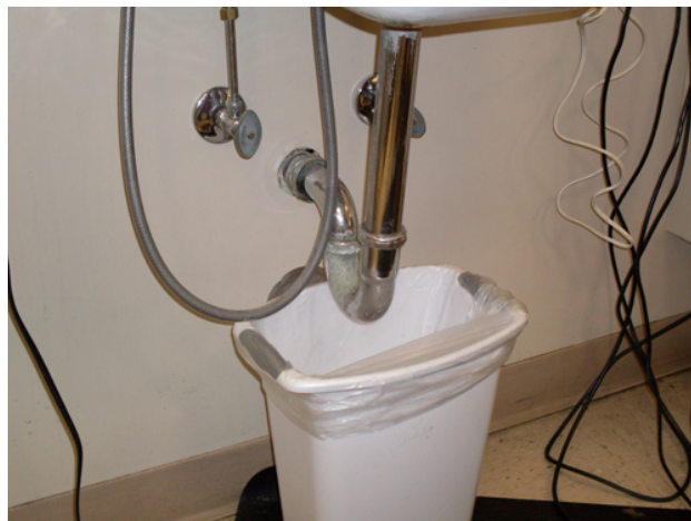
Figure 2. Photograph from the leaky drain problem-finding item.
