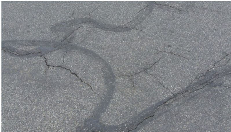
Figure 4. Photograph from the street cracks problem-finding item.
